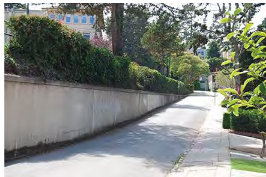
Example of one of the medians and retaining walls between divided streets.
