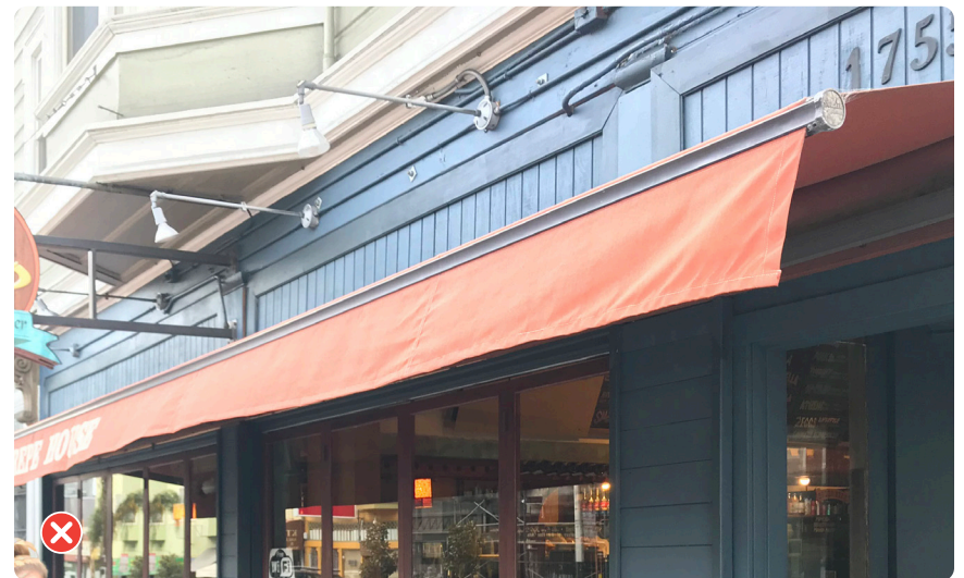
Inappropriate installation of gooseneck light fixtures
