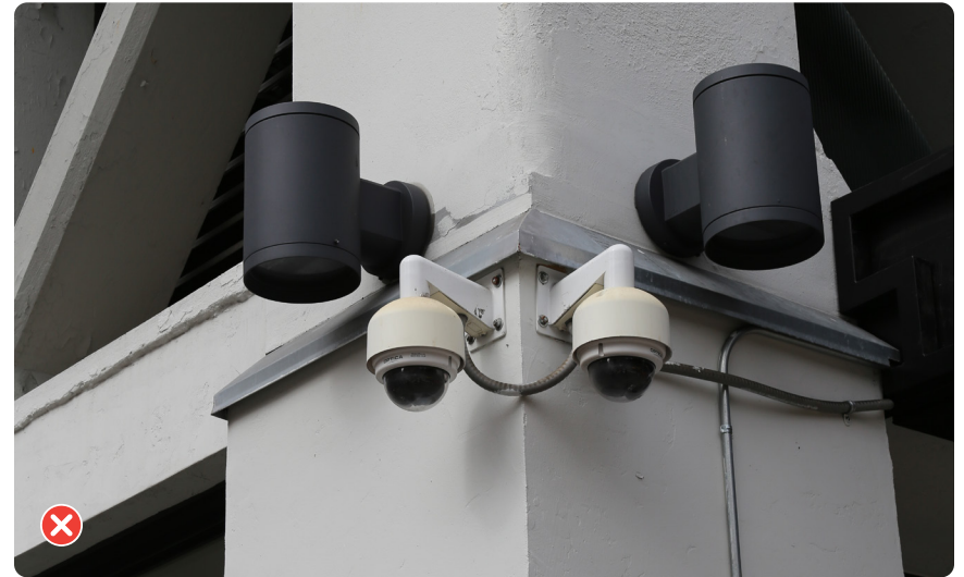
Security cameras installed with visible electrical conduit
