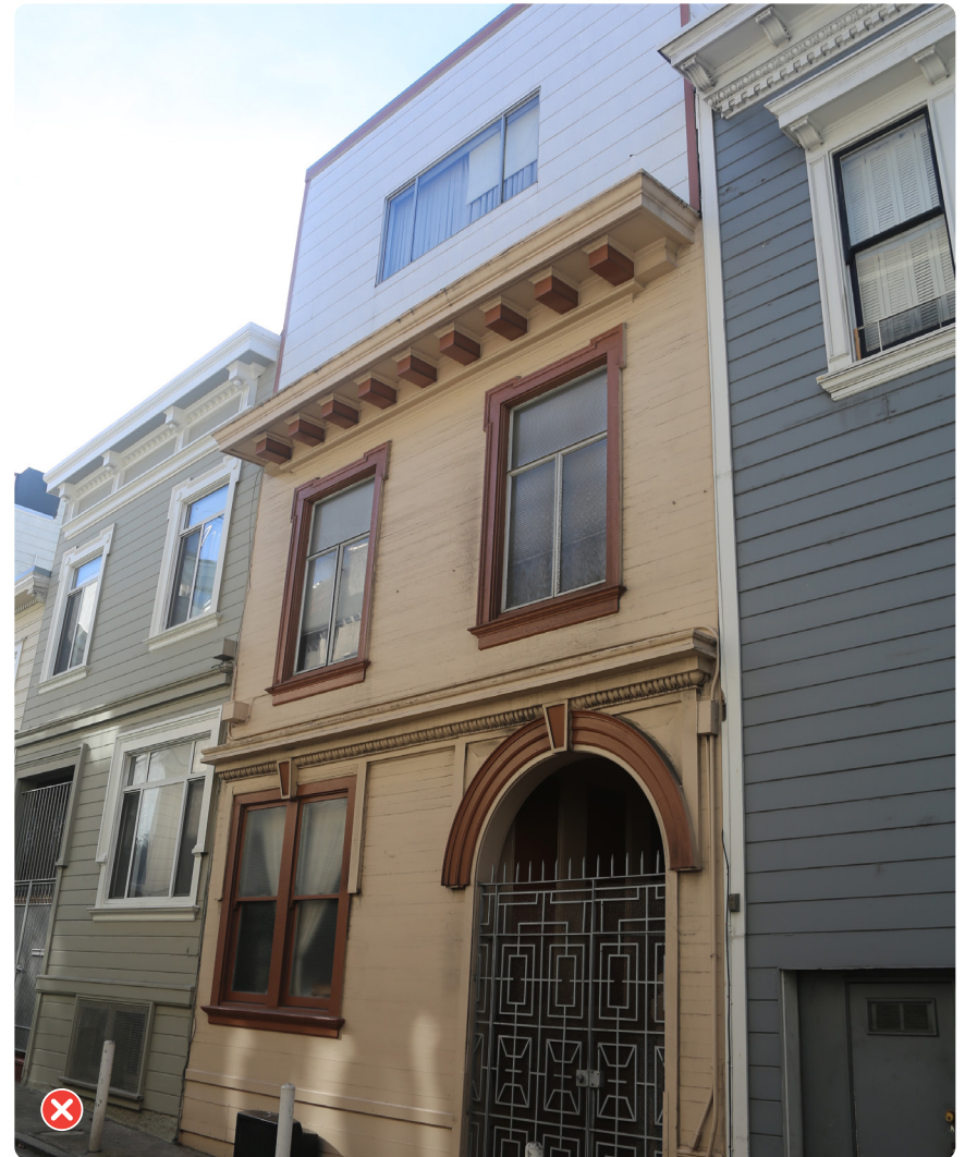
Inappropriate windows installed in an addition to a historic building that do not match the finish, operation, or material of the historic building's original windows
