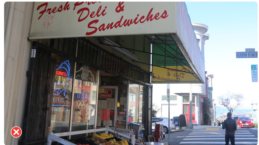
This waterfall awning is not installed in a window opening and covers character-defining features, overwhelming the historic storefront.
