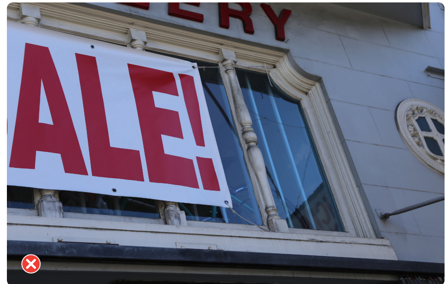
This signage covers up the character-defining historic storefront transom and does not meet Standard P.1.4.
