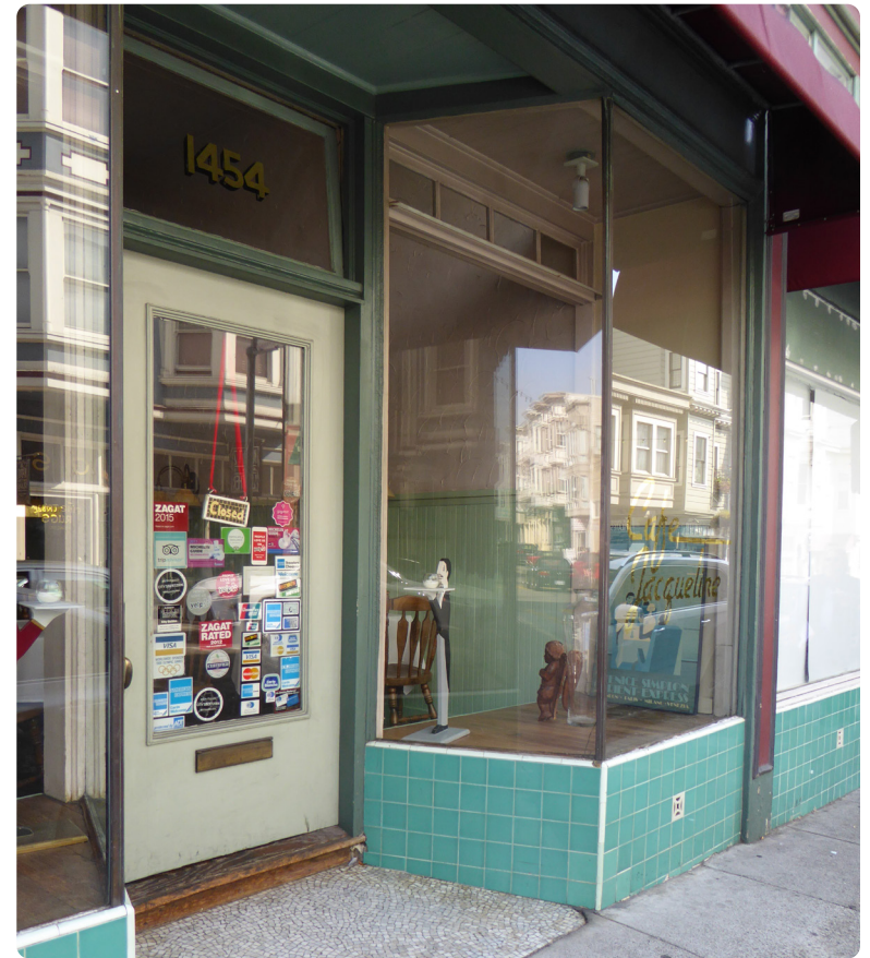
Historic storefront with tiled bulkhead, thin-profile storefront framing, recessed wood-and-glass entrance door and transom, and stone-tiled vestibule flooring
