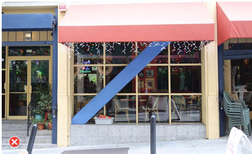
This seismic retrofit does not meet Standard P.7.3.1 due to its exterior diagonal bracing
