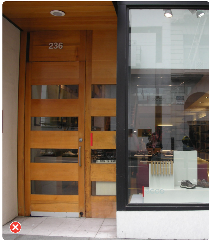
Incompatible replacement storefront door
